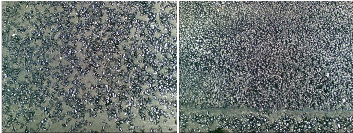
Figure 4.2 Newly laid surfacings on the TRL test track; HRA (left) and thin surfacing (right)
