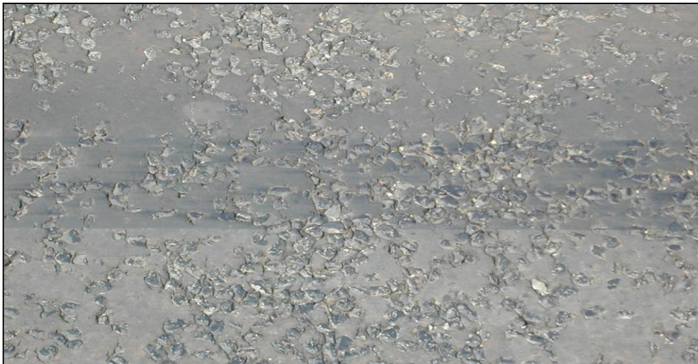
Figure 6.3 Skid mark from a dry PFT test on 1-month old HRA
